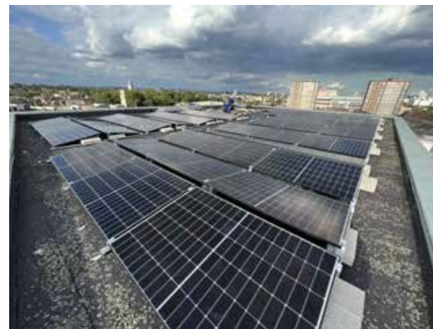
Example PV Panels.
