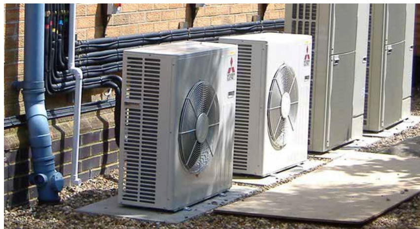
Example air source heat pump compressors.
